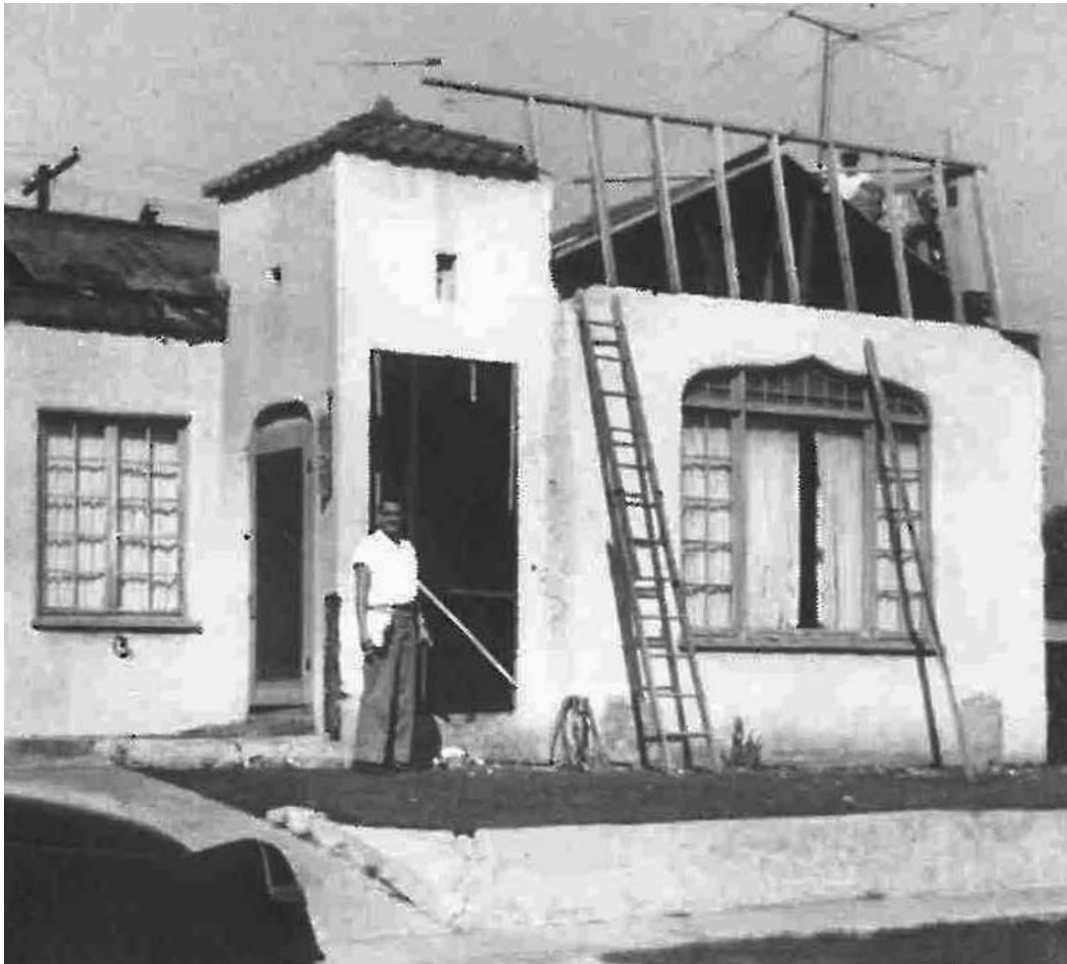
8937 Ashcroft Avenue in West Hollywood, remodeled by Larry Limotti and Ross Worsley in 1961–62. The framing for the mansard roof goes up on the 1920s bungalow. Photo by Larry Limotti.
